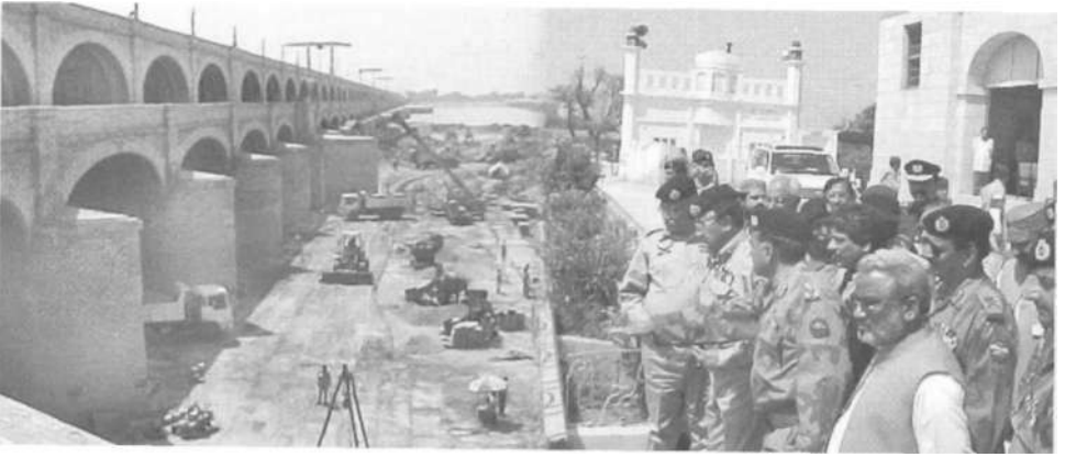
Inspecting the rehabilitation of the Sukkur Barrage, on the Indus River in Sindh
